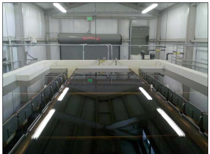
View from on top of the clarifier where the first step of treatment occurs. All equipment shown is new inside the new Worton WTP building.
